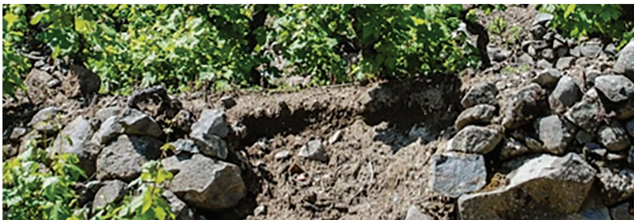
Collapsing drystone wall
