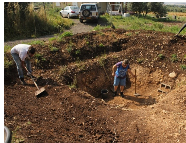
The team prepares the ground for the establishment of an ecological pond.
