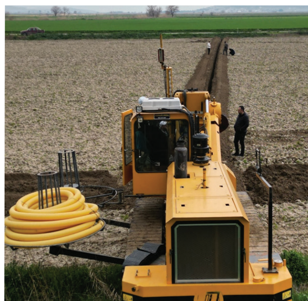
A view of the installation process of a subsurface drainage system using specialised machinery. The yellow drainage trencher is laying perforated pipes underground to improve soil conditions and prevent waterlogging and salinity problems in the field.
