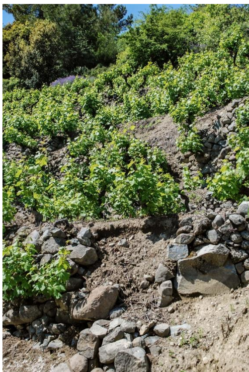
Figure 10: Collapsing drystone wall
