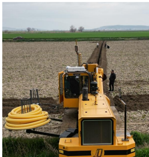
Figure 5: A view of the installation process of a subsurface drainage system using specialised machinery. The yellow drainage trencher is laying perforated pipes underground to improve soil conditions and prevent waterlogging and salinity problems in the field.
